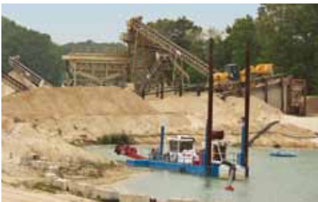
This dredge is responsible for deepening the original 80-year old sand pit an additional 30 feet. Note the 80Z7, ramp, and Grizzly separator in the back.
