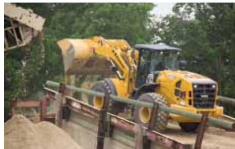
The wheel loader feeds gravel brought up by the dredge or long-reach excavator into their Grizzly separator.
